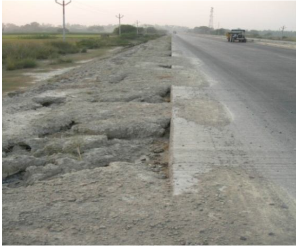
Photo-1 Severely Eroded Earthen Shoulder
