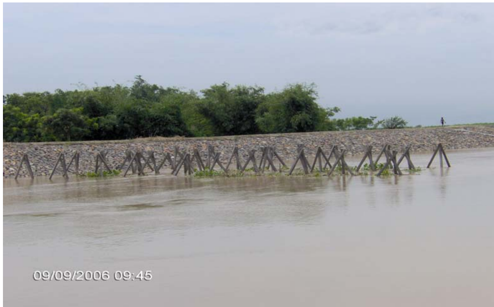
Fig. 5 showing one row of Porcupines used for bank protection upstream of Farraka barrage.
