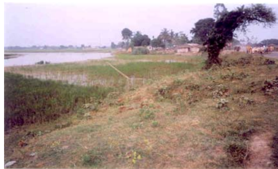
Fig. 17 Erosion on left bank of Bagmati River eroding the habitats U/S of bridge
