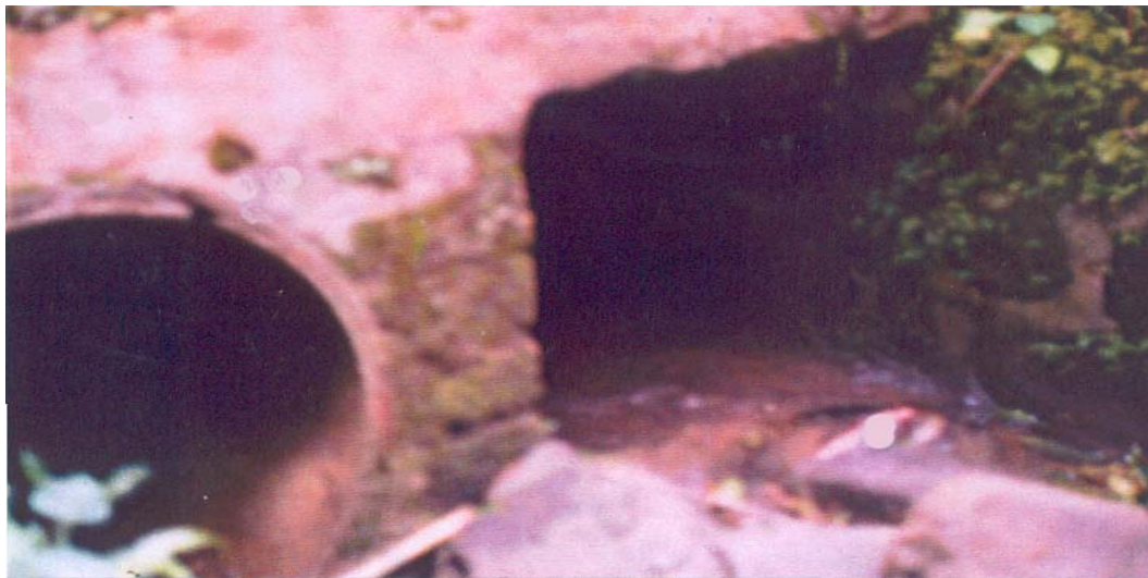
Photograph-4 (Showing a Box Type Culvert by the Side of a HP Culvert to Augment Flow Capacity)
