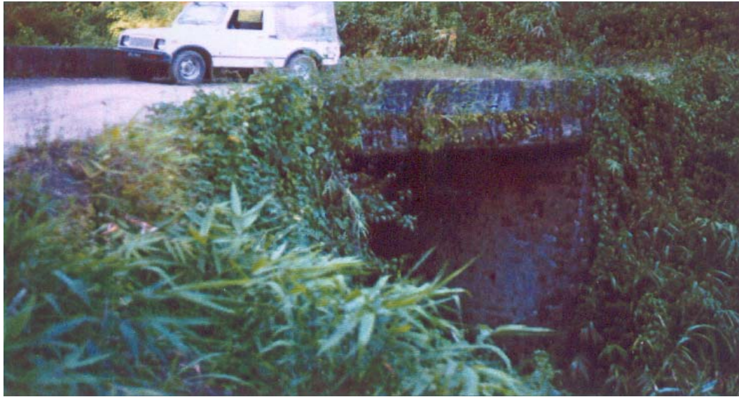
Photograph-3 (Showing Growth of Jungles Upstream of a Slab Culvert)
