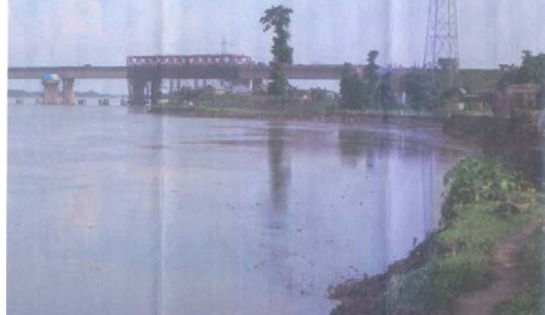
Fig. 9 Erosion on Right Bank of Mahananda River Showing Embayment U/S of the Bridge on NH-31 (Taken from Paper by Mazumder,2010)
