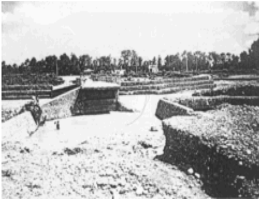
Fig. 7 Outflanking of a vented causeway on the stream 'Danab Khola' Bridge in Nepal
