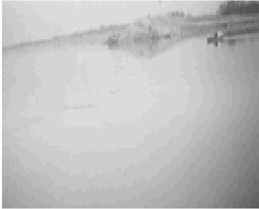
Fig.10 Washed Out Head of An Impervious Upstream of Farraka barrage
