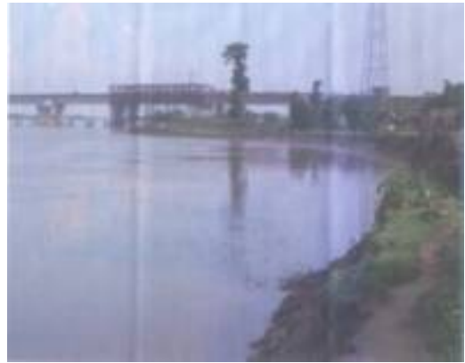
Fig. 8 Erosion on Right Bank of Mahananda River Showing Embayment U/S of the Bridge on NH-31
