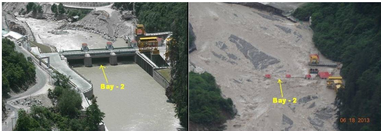
Photo.1 Aggradations of Alaknanda River Bed at Vishnuprayag HEP Barrage due to Landslides June, 2013 (Photos show bed levels before and After Flood). [Courtsey: S.D.Sharma, GMR Group of CO. New Delhi]
