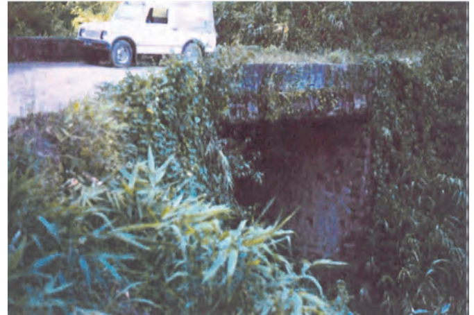
Photograph-4: Weed Growth near Culvert Inlet in a road in Mizoram
