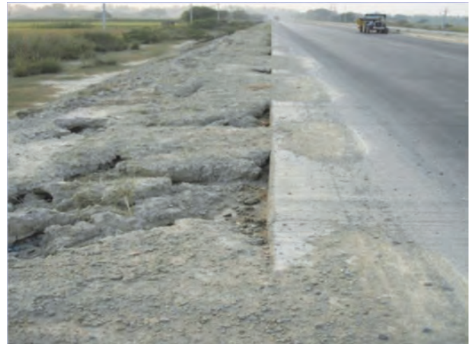
Photograph-1: Damage to Road Shoulders
