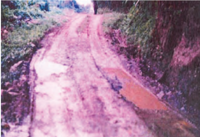
Photograph-3: Washing out of Pavement in a Hilly Road in Mizoram due to Improper Drainage
