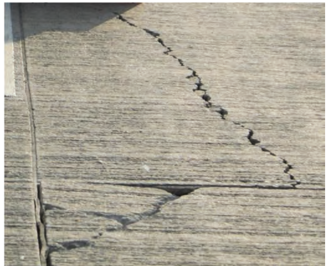
Photograph-2: Showing Crack in a rigid concrete pavement
