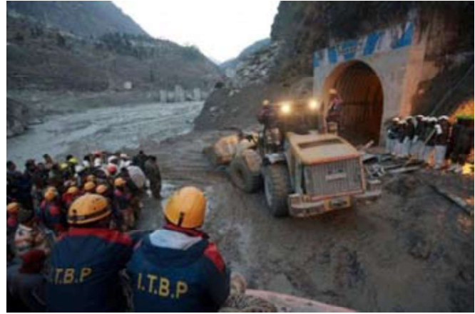
Fig.10 : National Disaster Response Force (NDRF) and Indo Tibetan Border Police (ITBP) search for workers trapped in a tunnel in Tapovan area on February7- 8, 2021.
