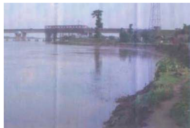
Fig.10 River Bank Erosion due to Anabranching of River Mahananda Upstream of Bridge on NH-34
